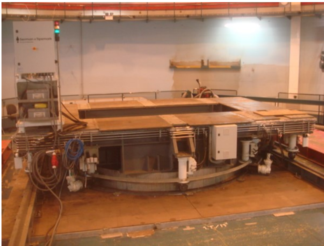
Figure 5. Movable Top Shield: a sliding platform enabling the reactor opening to be sealed after removal of the TSP. Photo courtesy of Danish Decommissioning.
