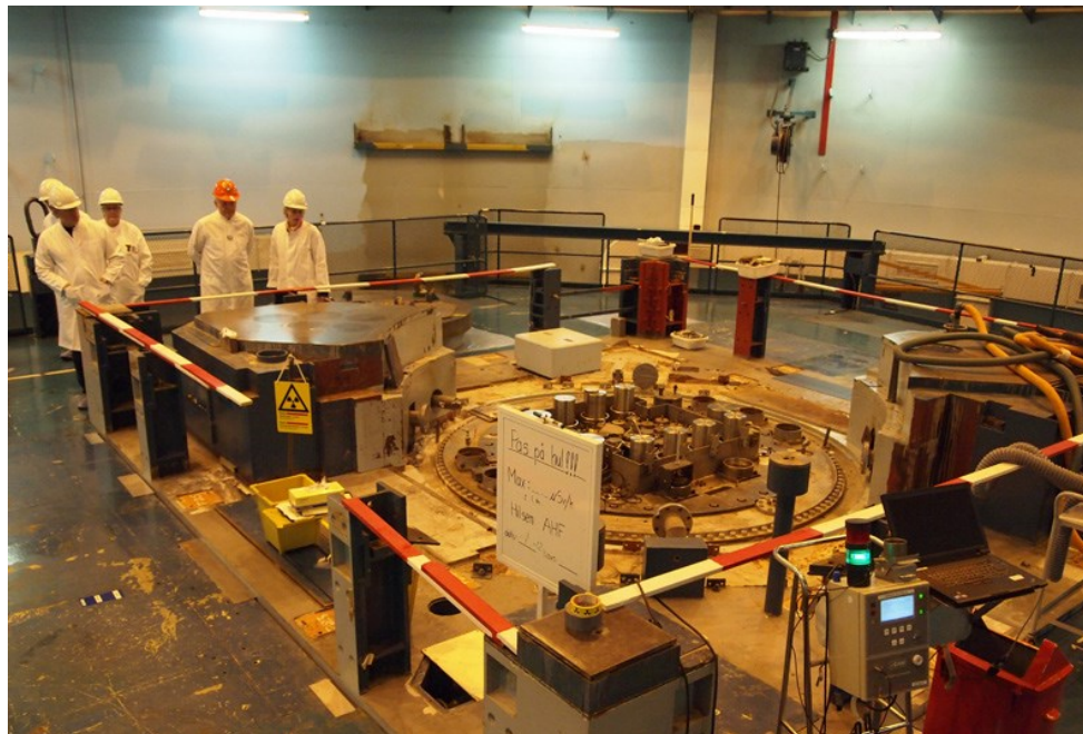
Figure 4. Top: Reactor top level. Master plane level is at the blue surface below in the picture. Bottom: Reactor top cleared to Master plane level with storage blocks still in place. Photo courtesy of Danish Decommissioning.
