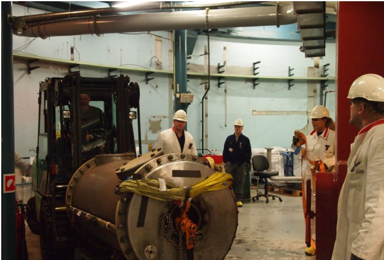
Figure 3. Removal of the last heat exchanger from the heavy water plant room. Photo courtesy of Danish Decommissioning.
