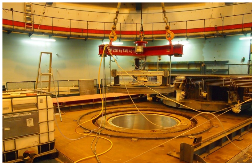
Figure 7. Lowering of the cutting equipment into the reactor opening prior to cutting of the RAT. The MTS with circular shielding plate is viewed in the background. Photo courtesy of Danish Decommissioning.
